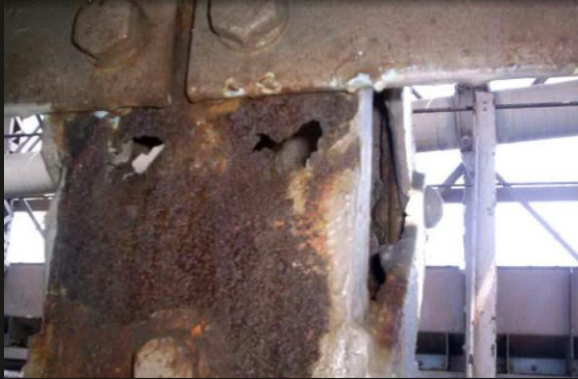
Holes in floor beams under the span from corrosion.
