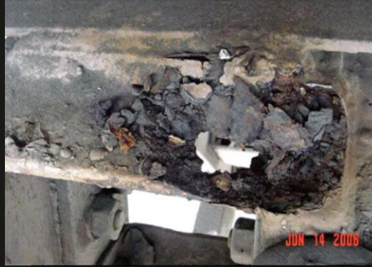
Corrosion on the base plate over floor beam.
