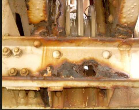
65% loss of steel on a floor beam due to corrosion.
