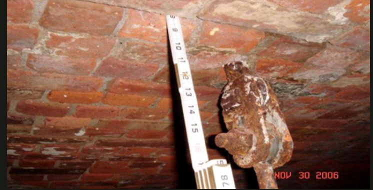
Ruler inserted 8 inches into a crack where Manhattan anchorage attaches to the span.
