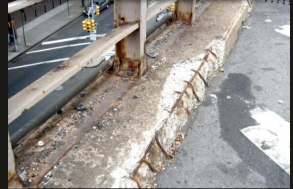
Exposed rebar on a curve on the Manhattan approach.
