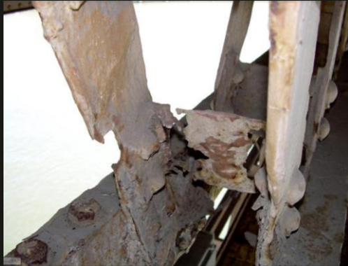
More corrosion of floor beams.
